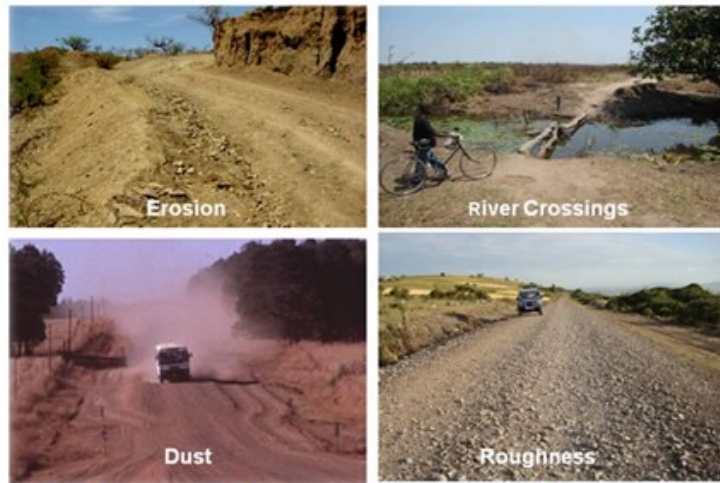
Typical problems on gravel road networks
